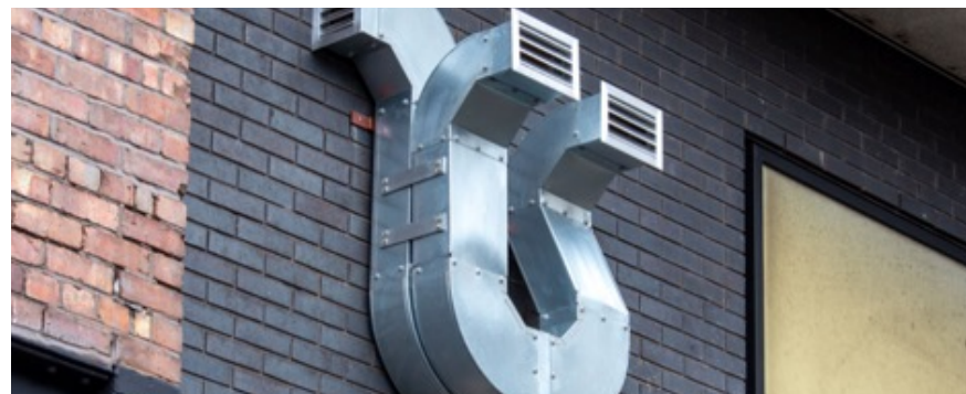
In the Image: Sparrow nests from twisted ducting
