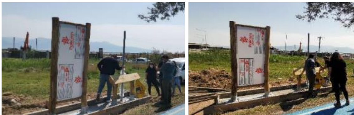
Figure 4-33: Implementation stage of information boards
