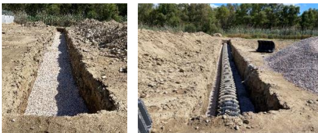
Figure 3-2: Excavation works and piping equipment implementation for grassed swales excavation work was started. Then, piping equipment of the drainage system was installed.
