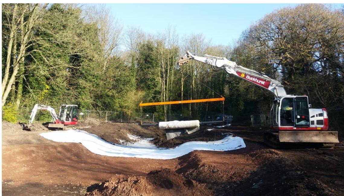
Figure 16: Onsite works at Otterspool water retention ponds. Laying the liner for the main pond.
